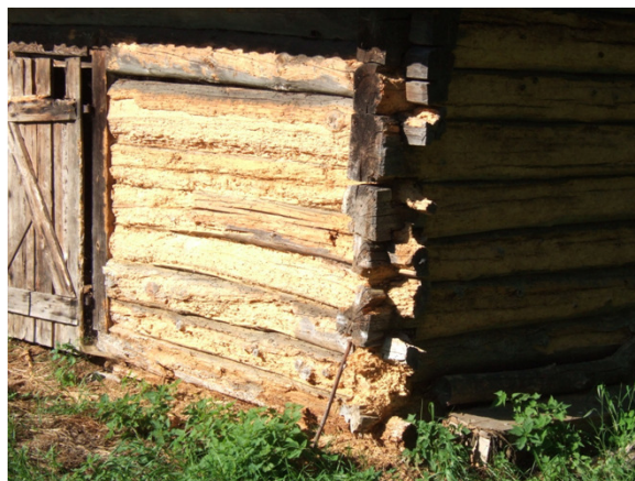
Corner of a barn Very heavy attack by Hylotrupes
