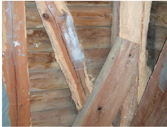
Severe attack in new church tower Strength reductions
