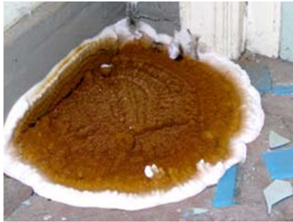
Dry rot fungus Not much of fungal attack
